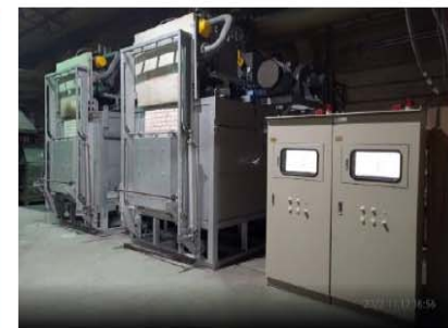
建置蓄熱式燒結爐
